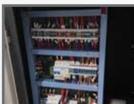
Industrial electrical Console
