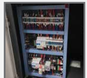
Industrial Electrical Console
